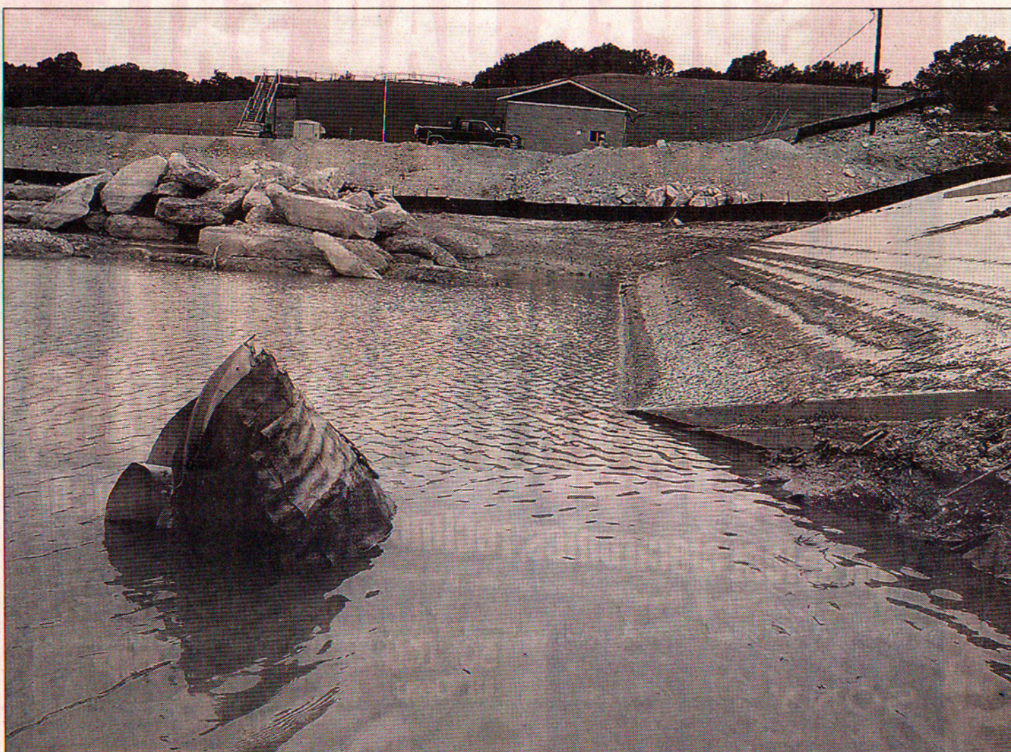
A drain pipe and filter, foreground left, in the detention pond at the West Cypress Hills development once kept runoff from getting into Lick
